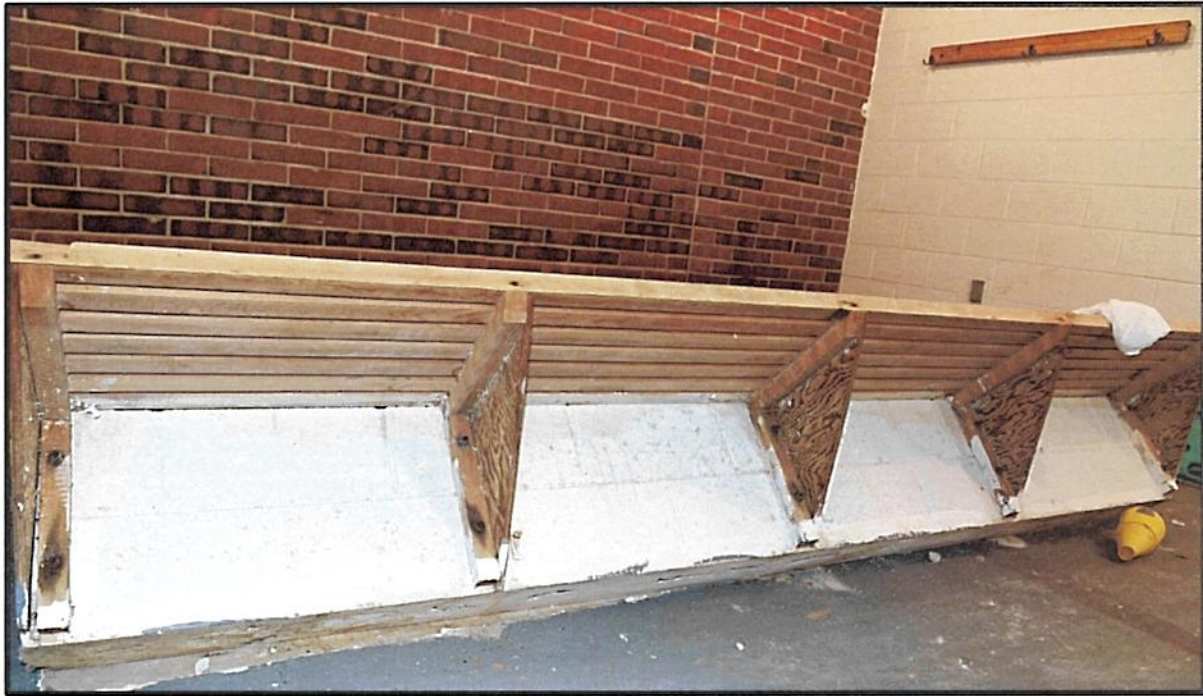
Figure 6.8: Partition Wall after Mishap (Tab Z-19)
