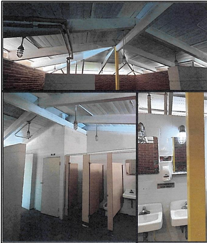
Figure 6.11 Mishap Site Lighting (Bathhouse Men's Side) (Tab Z-22)
