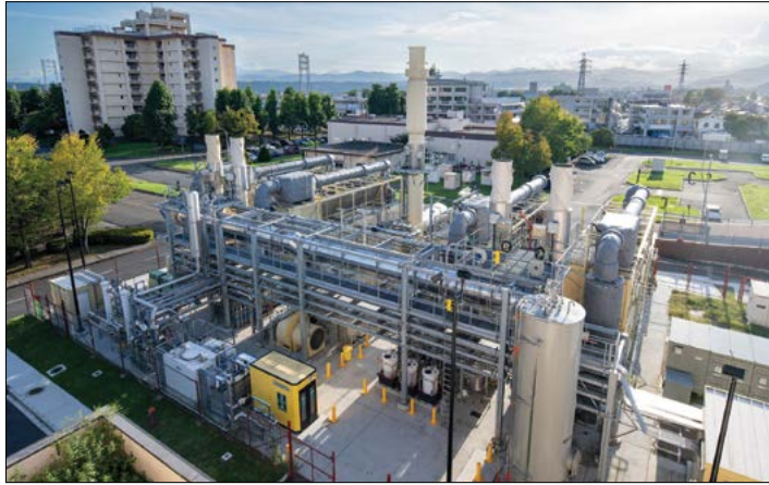
Photo courtesy Schneider Electric.
