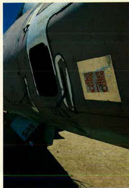
Although a Coke can is not the recommended material for repairing a shell hole, this ingenious fix shows how adept Aircraft Battle Damage Repair technicians are at using almost anything to get an airplane back into the flight.
