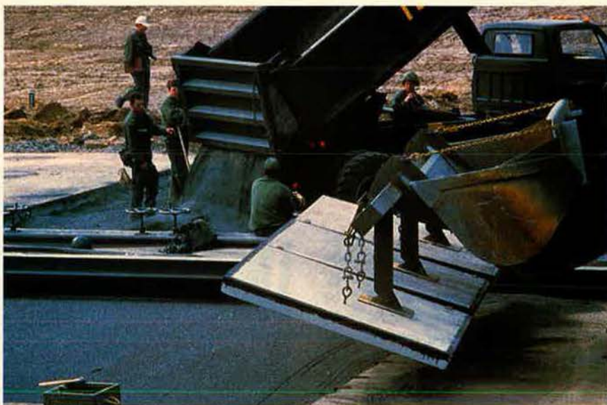
Maintenance crews perform rapid runway repair using a front-end loader to place concrete slabs. An essential offensive tool in "fighting the air base," runways are, naturally, a prime target. The more air base personnel are cross-trained to operate such equipment in an emergency, the faster an air base can recover from an attack.
