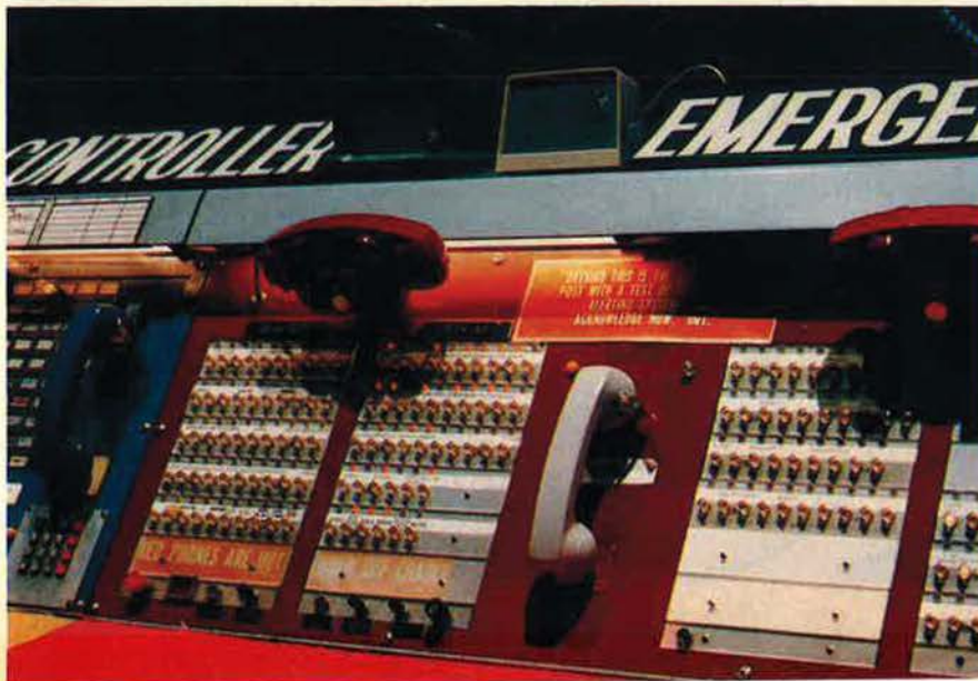
The red telephone in the underground command post activates the Primary Alerting System.
