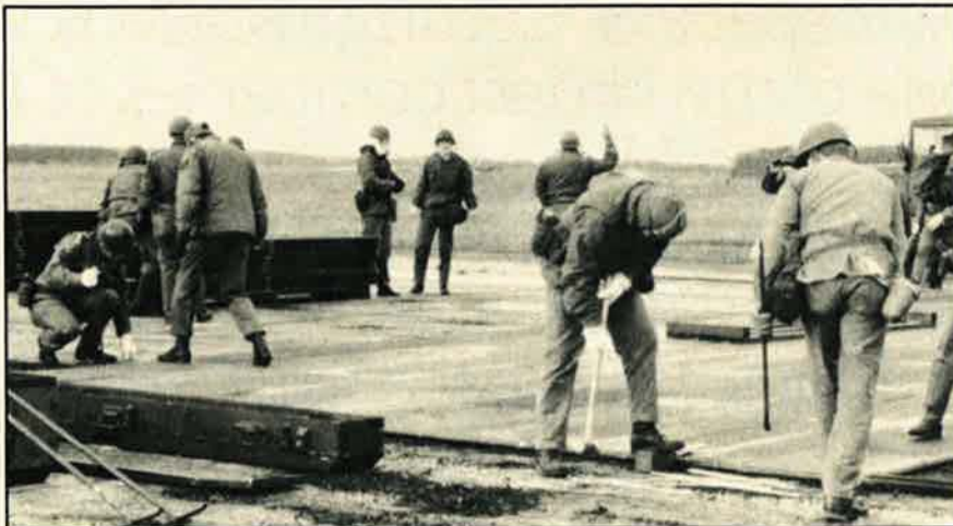
The RAF Bentwaters Rapid Runway Repair Team holds the UK record for laying a fifty-four-foot by seventy-seven-foot mat in sixteen minutes, nine seconds. USAFE is testing the use of concrete slabs instead of conventional aluminum matting as a quicker and more economical method of repairing runway craters.
