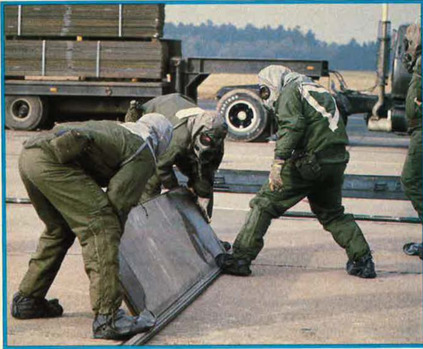
Civil engineers in full chemical ensemble practice rapid runway repair during an exercise at Hahn AB, Germany. A new technique for getting battle-damaged runways back into action employs concrete slabs instead of aluminum matting, a cheaper approach that requires less human labor.
