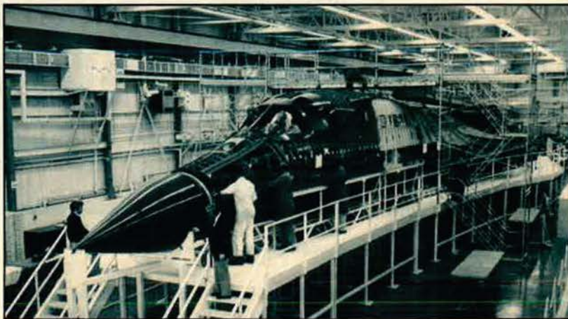
B-1B contractors are using the System Development Tool (SDT), located at Rockwell International's El Segundo, Calif., facility, to determine the exact route of wires, coaxial cables, and tubes that will go into the bomber.
