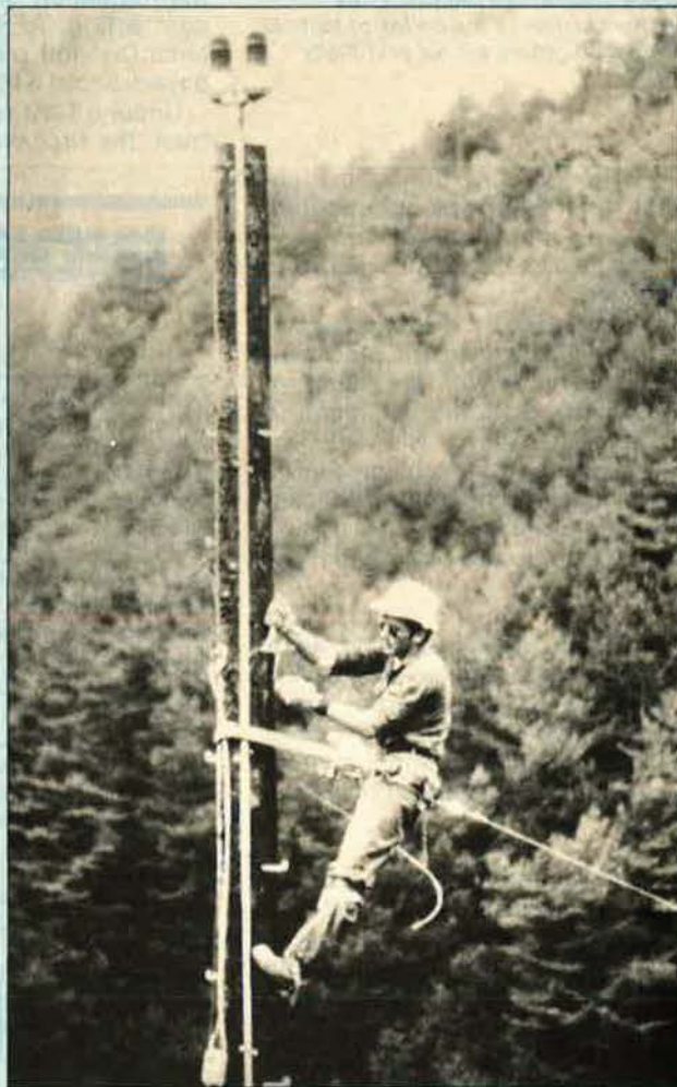
Sgt. Robert Foley installing a high frequency antenna during construction of the Korean Tactical Range, KOTAR. (USAF photo by TSgt. Bertram W. I. Mau)
