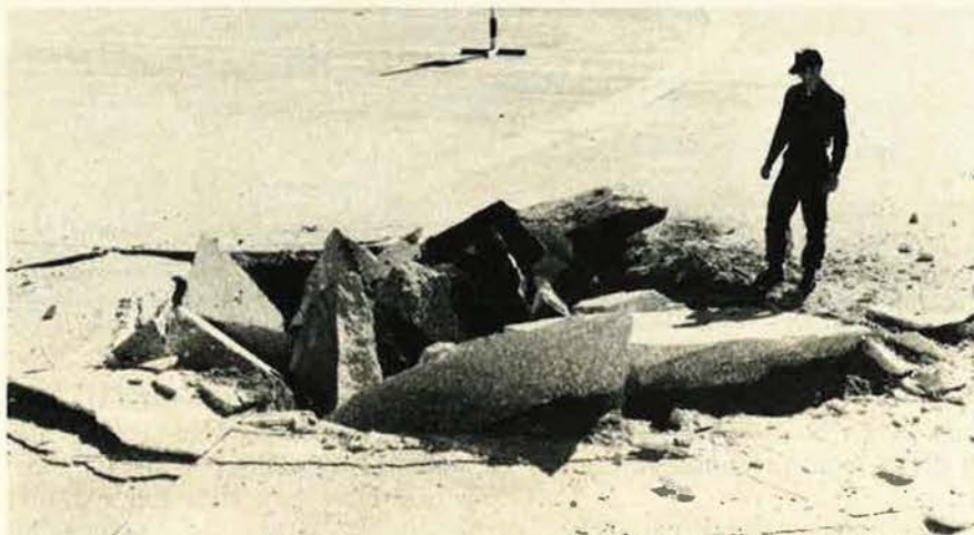
What a pothole! Crater in test taxiway at Eglin AFB, Fla., shows the dimensions of the rapid runway repair challenge being met by USAF's Civil Engineering Center. The object is fast repairs to restore forward bases to sortie-launching service.
