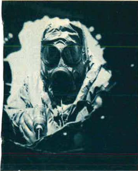
Electrician SSgt. Henry Ware, 2955th Combat Logistics Support Squadron, drills holes before installing a "scab" patch on an F-105. (USAF photo by TSgt. Dave Bowers)
