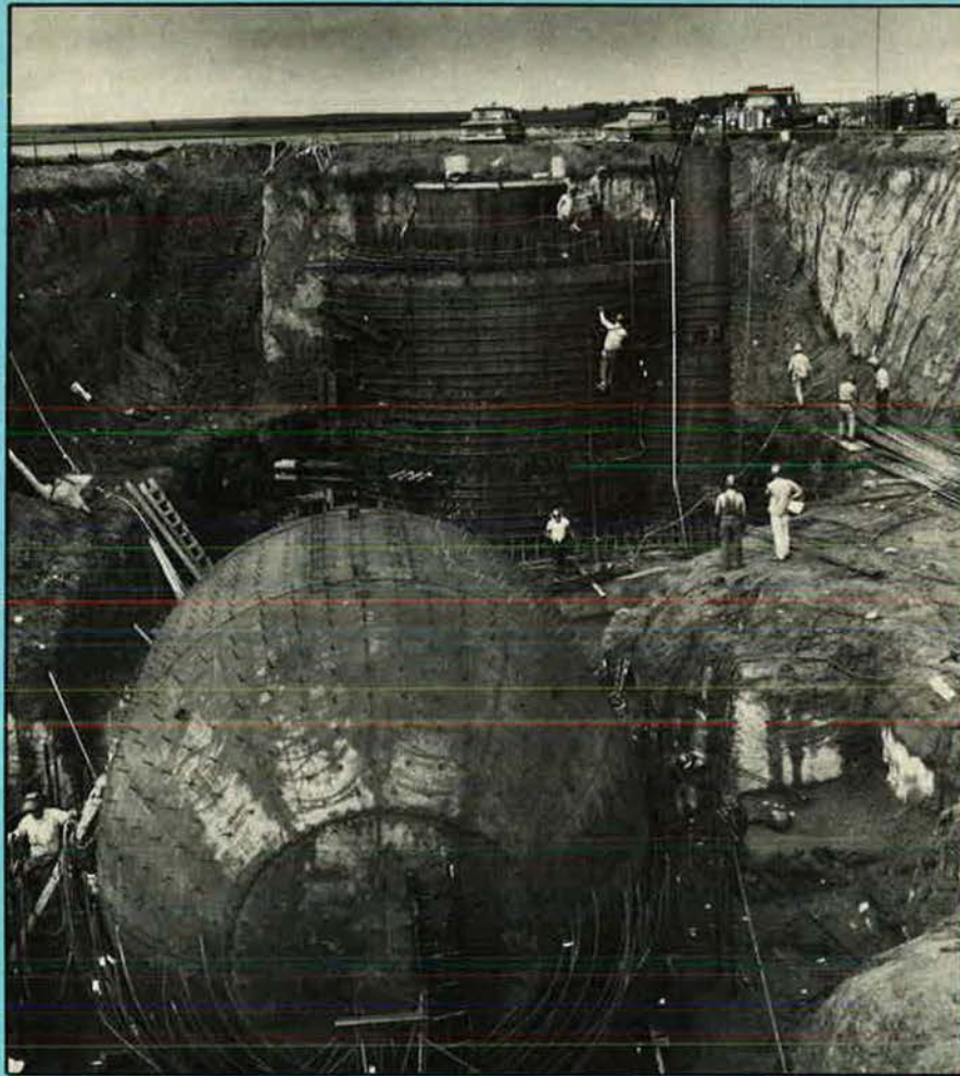
Designing and constructing the hardened facilities for 1,054 ICBMs was one of the greatest engineering feats of history. In the foreground of this Minuteman site is the equipment building, with the missile silo in the background.
