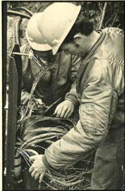
Members of Maine ANG's 243d Electronics Installation Squadron splice a cable at Loring AFB, Me.
