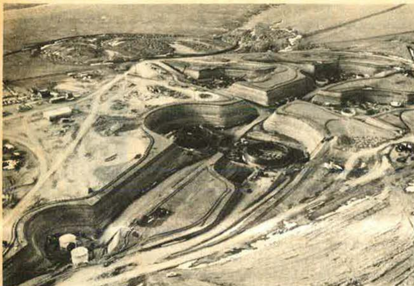
Building a Titan ballistic missile complex, such as the one shown here, entailed massive construction and earthmoving efforts. Different from Minuteman systems, the Titan silo and launch control center are collocated.
