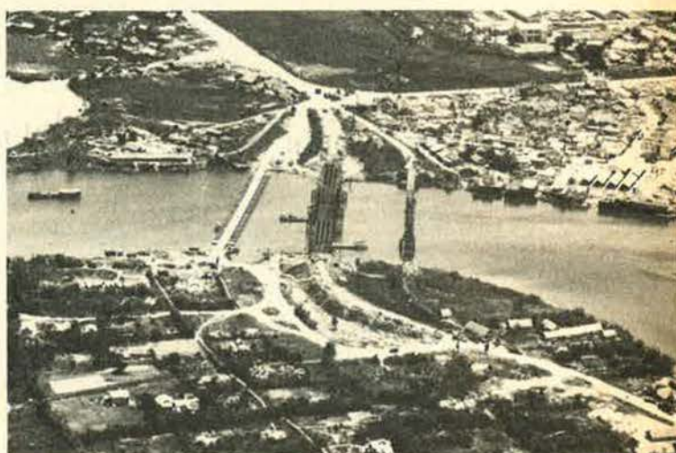
Dong Ha bridges under construction in August (top). By December the highway bridge was nearly completed.
