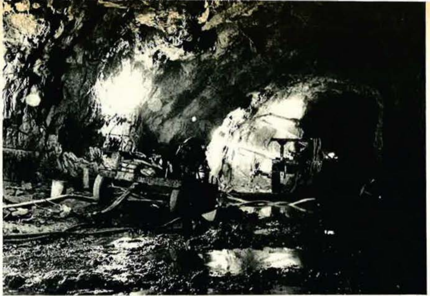
Cheyenne Mountain near Colorado Springs, Colo., will soon house a new utilities plant for the NORAD underground command post. Another phase of the modernization program will be construction of a control center for the Safeguard antiballistic missile system.
