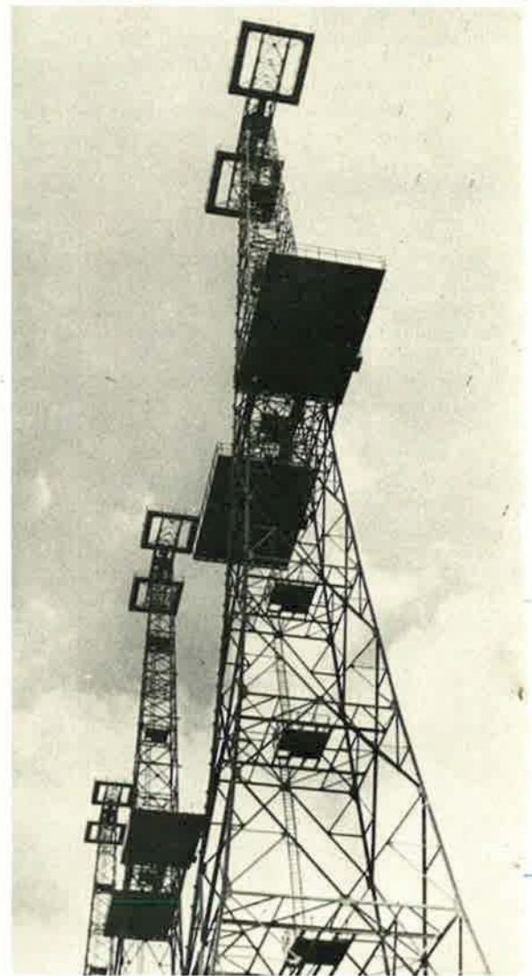
The British were the first to get an operational radar system to the field. These 360-foot-high masts were part of the radar net that was instrumental in winning the Battle of Britain.
