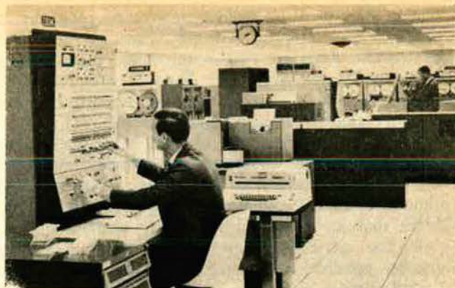
The Seventh Air Force's Seek Data II command and control system employs a standard, commercial computer, the IBM 360/50, as shown here. The Air Force uses commercially developed, general-purpose systems when possible to cut costs.
