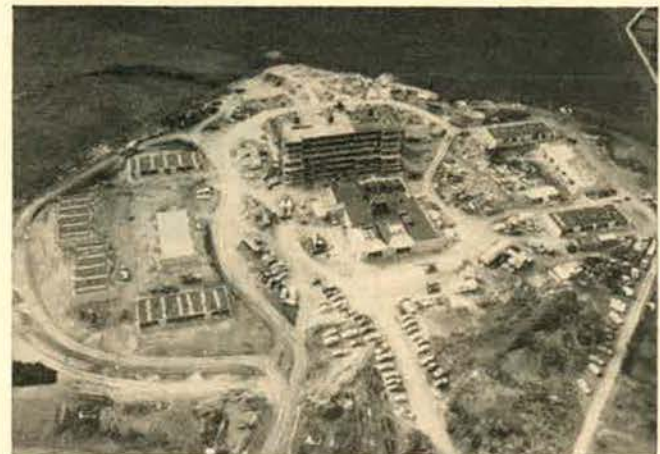
Since ground was broken for Air Force Village last May (see July 1969 AF/SD, page 22), work has gone right along on the project. Shown here, in a photo taken late in 1969, is a panoramic view of the partially completed Village—the high-rise, garden apartments, and shopping center. As a retirement home for USAF career officers, their widows and dependents, the Village, which will include a community center and health and recreation facilities, should be ready for occupancy late this year.
