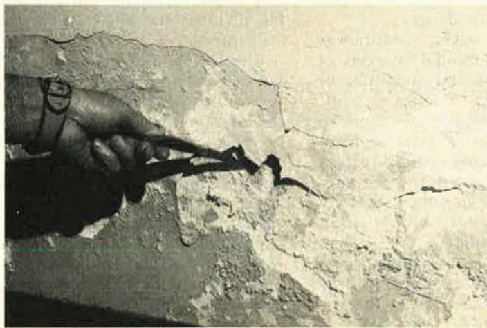
Moisture damaged this BOQ wall at Mather AFB, Calif. Delaying repairs such as this increases their average costs by three percent each year.
