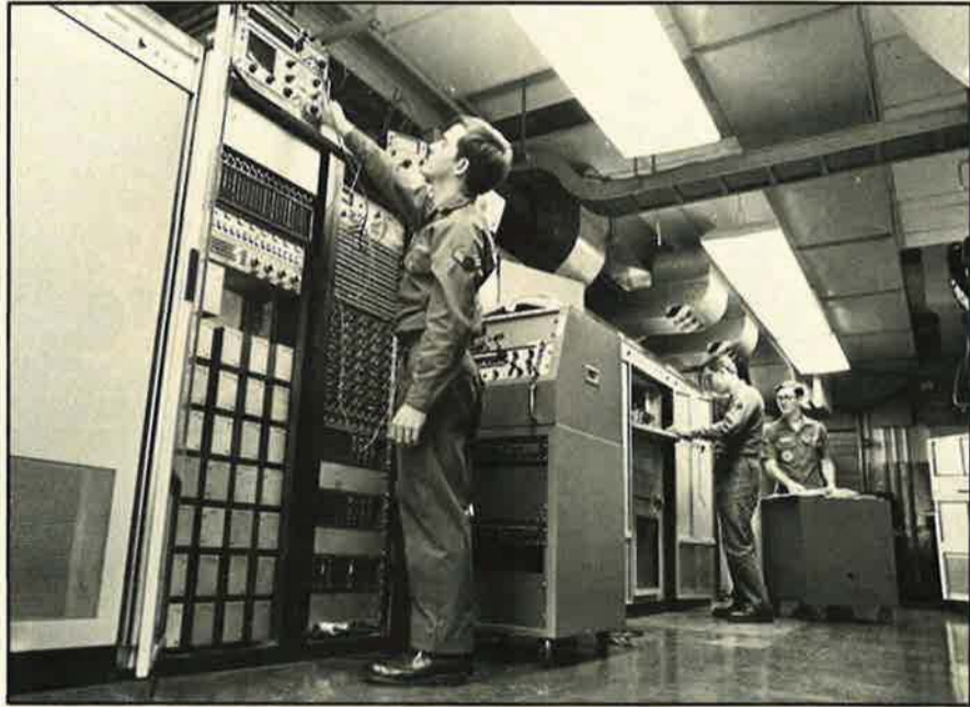
Technicians make preventive maintenance checks at the 1974th Communications Group's aeronautical radio station outside Scott AFB, Ill.
