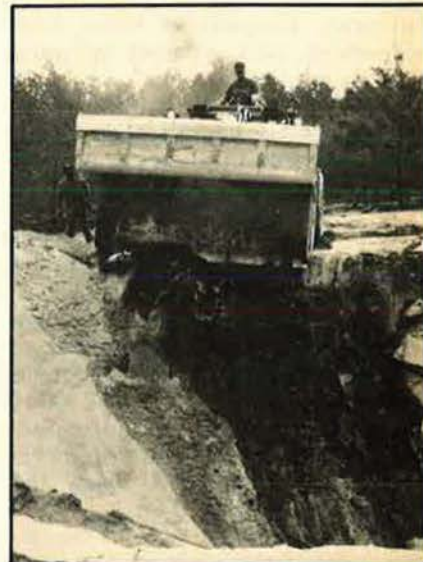
AFESC is advancing the technology for rapid repair of runways, and for quick recovery after bomb damage.
