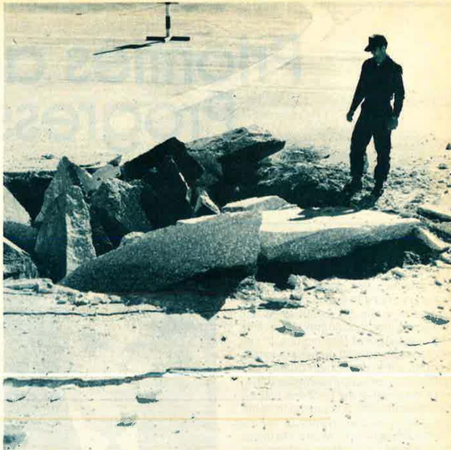
Runway damage caused by Matra Durandal test at Armament Division, Eglin AFB, Fla.
