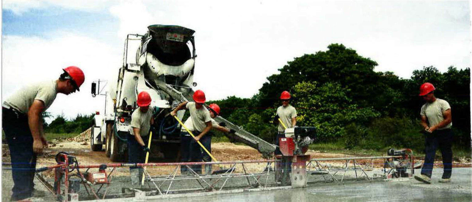
RED HORSE airmen float concrete at a runway training area on Guam. USAF has been moving toward a crater-filling method called flowable fill.
