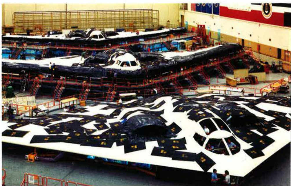
B-2s under construction at Northrop's Pico Rivera plant in California. The facility was subjected to the highest security measures.
