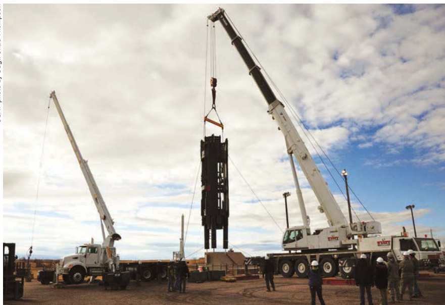
Left: A 47,000-pound missile support system is hoisted out of a launch training facility at Warren. While it's being repaired and refurbished, maintainers will perform corrosion control and other preventive maintenance in the silo. Below: An inert Minuteman III ICBM is lofted into space from Vandenberg AFB, Calif. Minuteman missiles are being upgraded and modernized.
