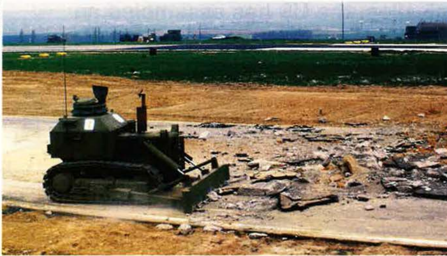
An armored bulldozer clears debris and live ordnance from the runway after one bombing run during the base survivability exercise.
