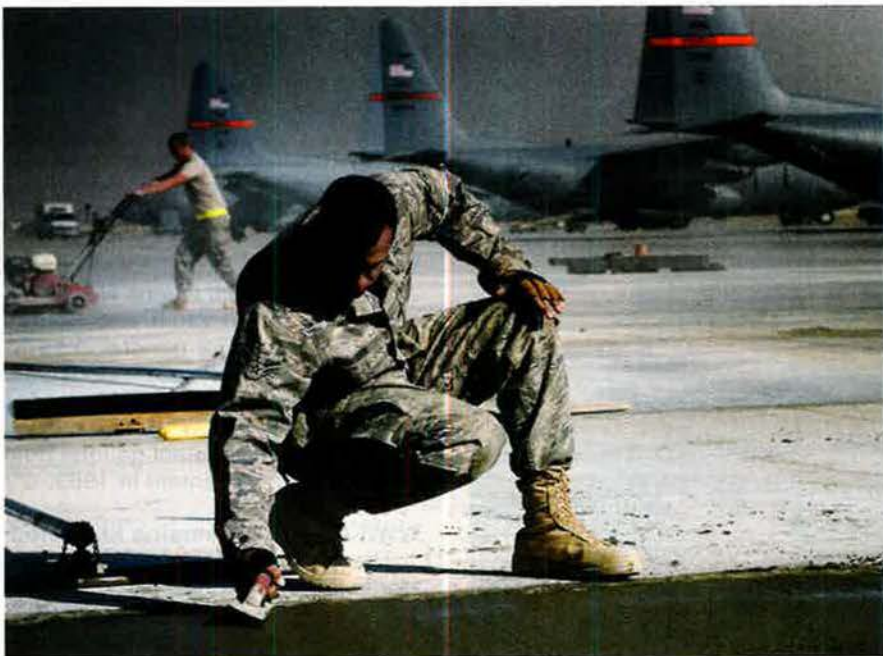
Making It Permanent: A1C Joshua Toth smooths wet concrete at Bagram Airfield, Afghanistan. Toth is a heavy equipment operator with the 455th Expeditionary Civil Engineer Squadron. There are 25 active construction projects under way at Bagram.
