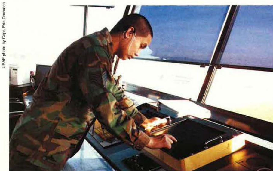
SSgt. Mark Paraoan monitors the lighting control panel of the new instrument landing system at Ramstein AB, Germany. Three days after going operational on Dec. 22, it allowed a C-17 loaded with patients from Iraq to land safely in poor visibility conditions.
