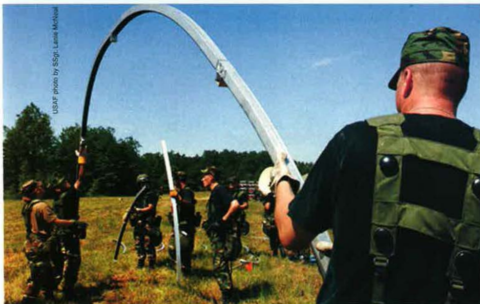
Airmen with the "421st Air Expeditionary Group" begin constructing small shelter tents used to house troops during an Eagle Flag exercise.
