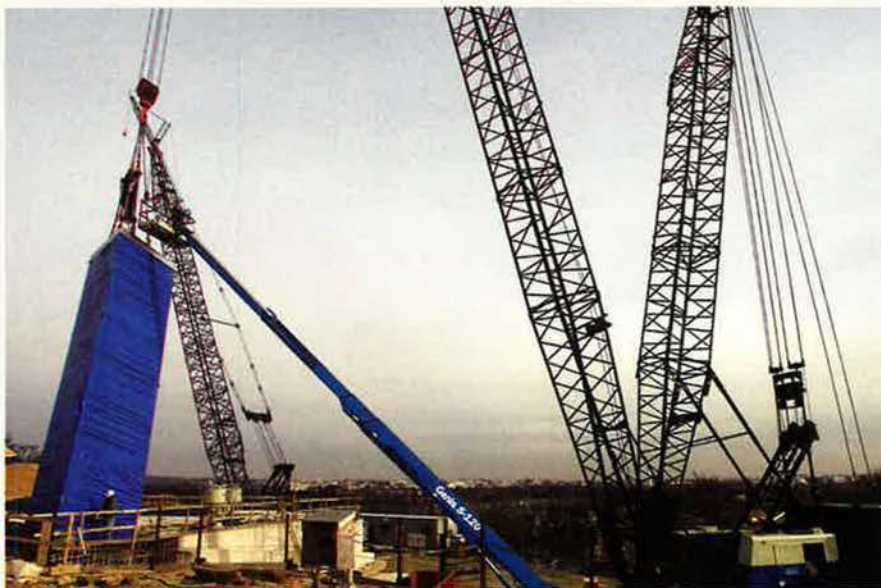
The first 39-foot section of a 279-foot-high spire—one of three tall structures that will comprise the Air Force Memorial—was set into place Feb. 10 at the memorial site near Arlington National Cemetery. Dedication ceremonies are scheduled for the fall.
