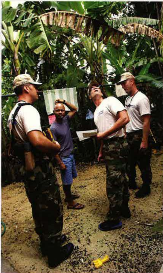
A civic action team composed of 13 airmen is working in the Pacific Island nation of Palau, where they have finished building an emergency search and rescue station, built a pavilion for Palau Community College, and repaired roads and schools. At left, TSgts. Jamle Pahukoa, Dave Vlnatleri, and Mike Luhmann discuss an upcoming project with a Palauan during a visit to a Head Start program facility.
