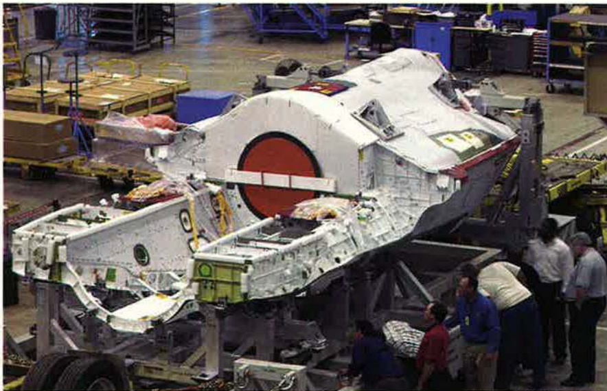
Lockheed Martin is assembling the first flying F-35 in Fort Worth, Tex. Above is the Northrop Grumman-built center fuselage, which arrived in Texas on May 3. It will be joined to a Lockheed-built forward fuselage and a BAE Systems aft fuselage.
