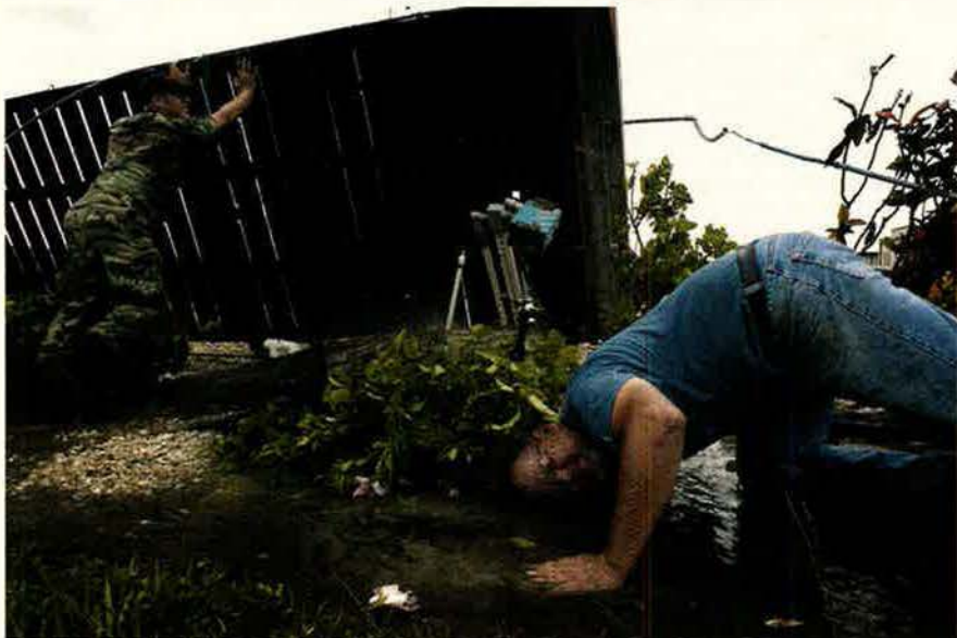
Phil Hyde (foreground) reaches to shut off a broken water line at Patrick AFB, Fla., following Hurricane Frances. Hyde, a plumber with the 45th Civil Engineer Squadron, was part of the initial recovery team.
