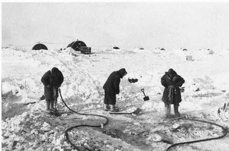
Paging Nanook. Construction workers drill foundation piers for a DEW Line building on Canada’s Baffin Island, north of the Arctic Circle. Temperatures at such sites could hit 65 degrees below zero.
