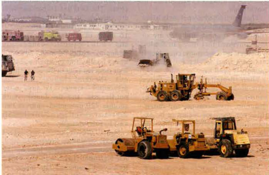
Members of the 823rd RED HORSE level an area of the desert in preparation for a new aircraft parking ramp. The region's harsh conditions make the engineering unit's job a particular challenge.
