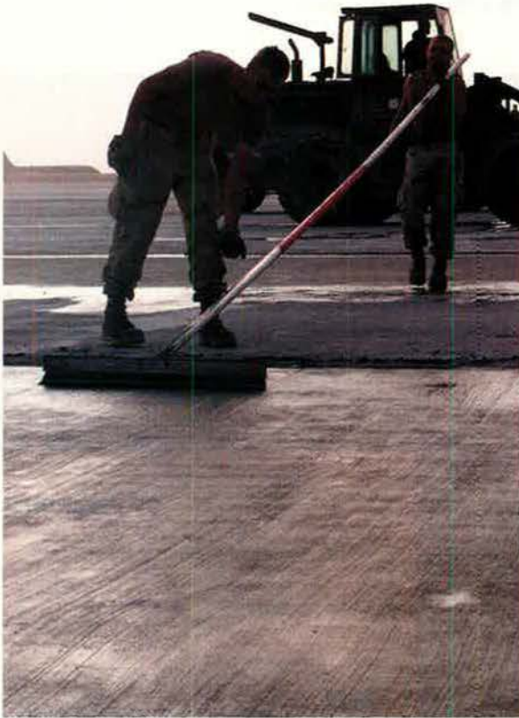
At al Udeid air base in Qatar, 823rd RED HORSE Squadron members apply the finishing touches to the concrete surface of a new 1,240-foot ramp. USAF civil engineers did everything from preparing the ground to obtaining fill materials to pouring and shaping the concrete.
