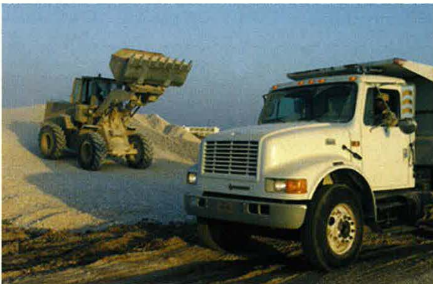
It takes some work to build a base from scratch. SSgt. LeRoy Huyghue III waits in his dump truck for TSgt. Dale Scott to deposit a load of gravel destined for a tent city the 823rd RED HORSE Squadron is creating at a forward location.
