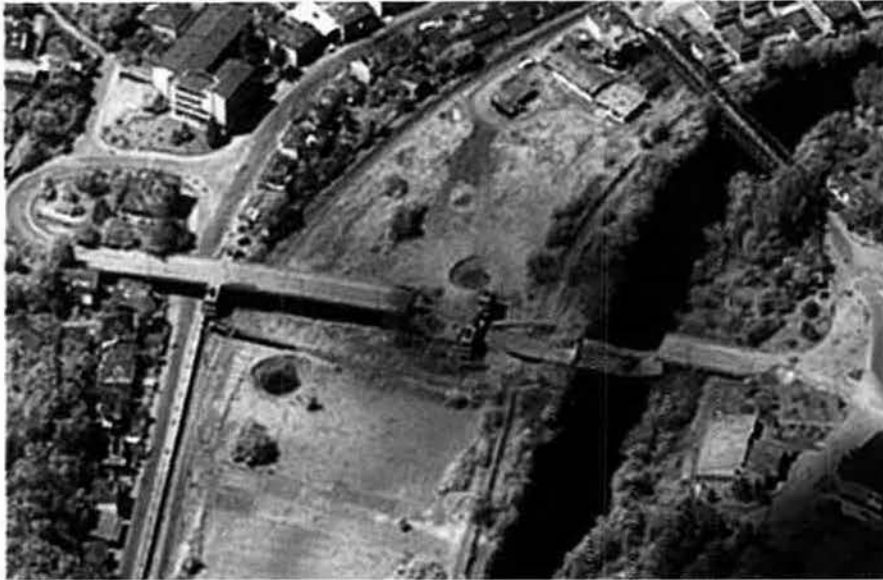
A damage assessment photo of a bridge in Serbia shows that a span was hit during precision bombing. For this type target, greater precision is gained at higher altitude.
