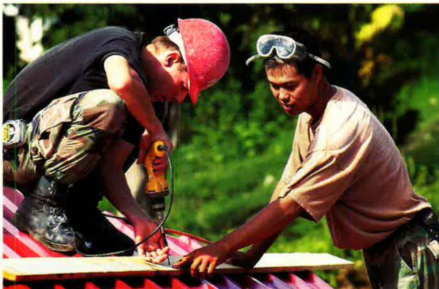
A1C Jerrod Roe (left) and SSgt. Ronalto Mactal, both from the 820th RED HORSE Squadron, Nellis AFB, Nev., work on the roof of a community center in Grenada in July. The squadron and a Marine battalion were supporting a US Southern Command humanitarian exercise, New Horizons 2000.
