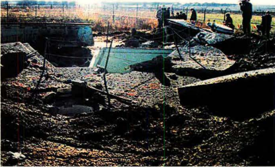
The implosion of a site called Hotel-11 marked the end of the last Minuteman II missile silo to be destroyed under terms of the 1991 START I accord. Located near Dederick, Mo., H-11 had been under the 351st Missile Wing's command.
