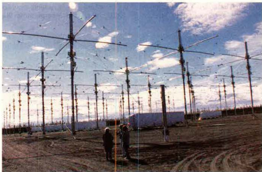
Alaskan residents view progress on the USAF-Navy High-frequency Active Auroral Research Program, which ultimately will feature 180 70-foot-high antenna towers spaced at 80-foot intervals in a rectangular grid—designed to research space weather effects—located at Gakona, Alaska.
