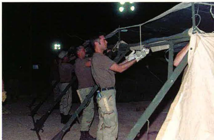
At first, USAF RED HORSE units did most of the heavy lifting. They handled the equivalent of 25 C-5 loads of lumber, canvas, generators, and other supplies so that arriving troops would have places to eat, sleep, and do their work.
