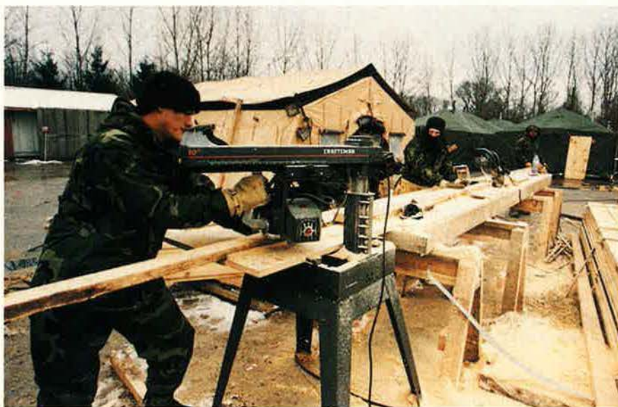
Colonel Waylett is proud of the RED HORSE crew, who, despite the lack of the customary lead time to plan for the deployment, have “stepped forward and met every challenge.”
