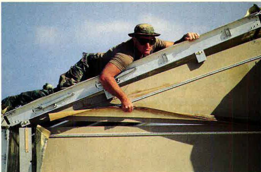
Deployments to remote regions hinge on specialists skilled in setting up support infrastructure, turning bare bases into operating bases with water, shelter, and other necessities. Here, a 366th Wing civil engineer builds a barracks in Egypt.
