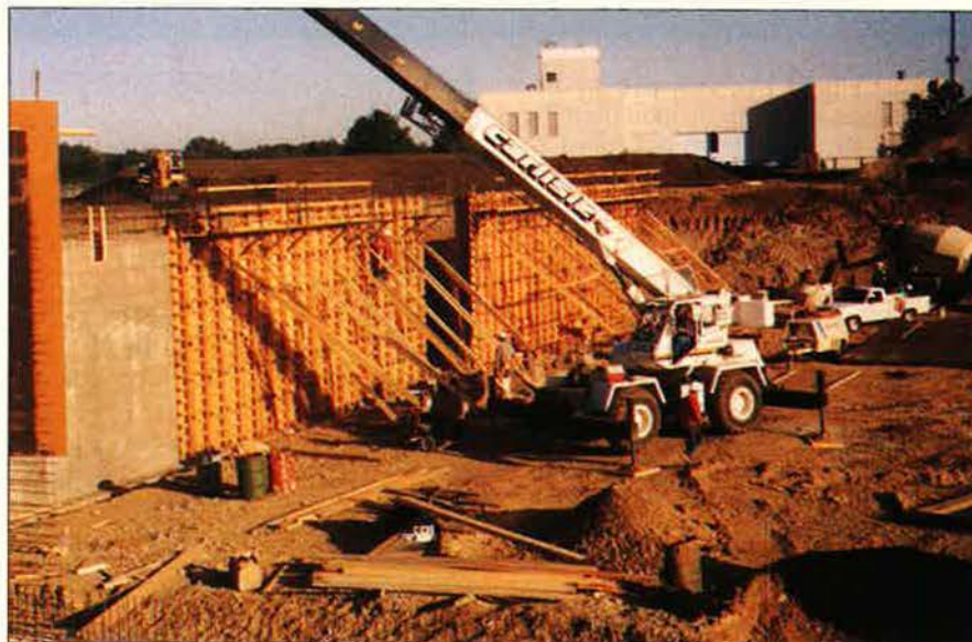
Construction continues on the new acquisition management center for Air Force Materiel Command's Aeronautical System Center. Work is expected to be completed by late March 1994. The project, commonly known as ASC Tomorrow, will be located just east of the Air Force Museum at Wright-Patterson AFB, Ohio.
