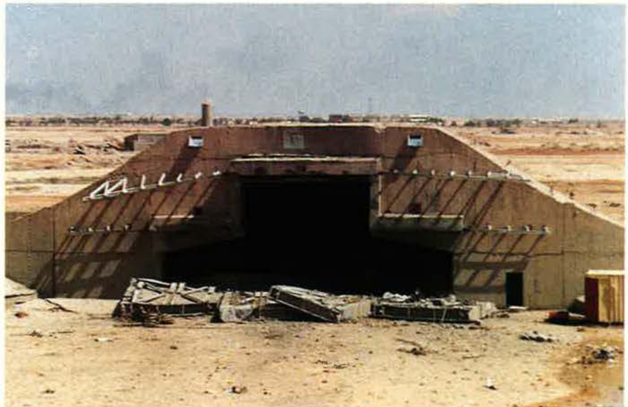
Precision weapons struck this hardened aircraft shelter at Tallil AB, Iraq, blowing out its concrete doors and charring the interior. The Air Force attacked most of Iraq's 600 or so hardened aircraft shelters, destroying or badly damaging at least 375 and probably destroying at least 140 aircraft.
