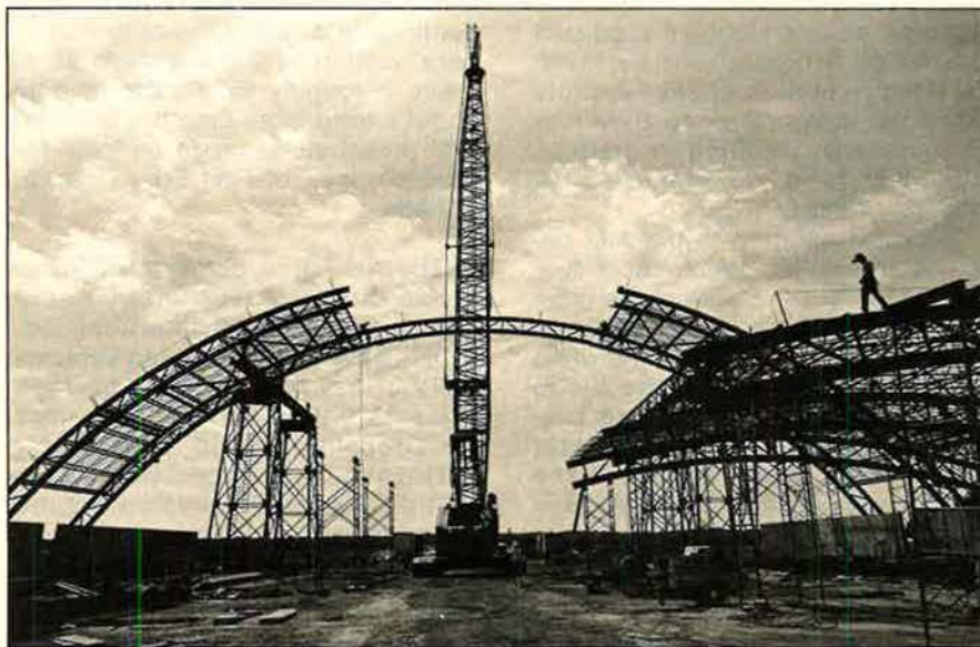
The first roof arch for the new $10.6 million addition to the USAF Museum at Wright-Patterson AFB, Ohio, was recently put into place. When completed next year, the addition will double the size of the Museum. (USAF Museum photo by Harry Elliott)
