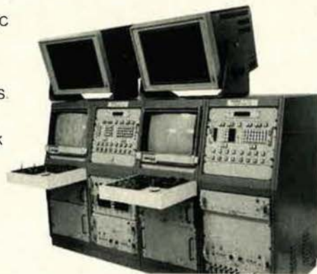
AN/FPQ-18 COMMAND AND CONTROL CONSOLE
