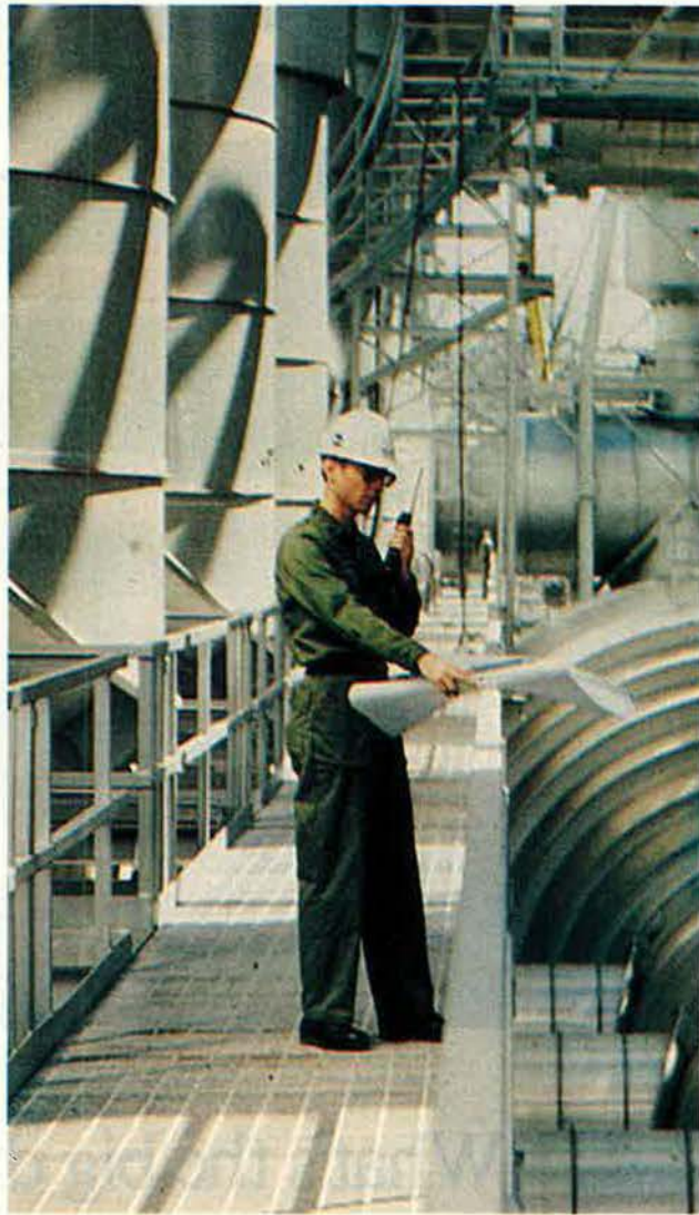
An engineer inspects the Aeropropulsion Systems Test Facility (ASTF) exhaust ducting as part of shakedown activities.
