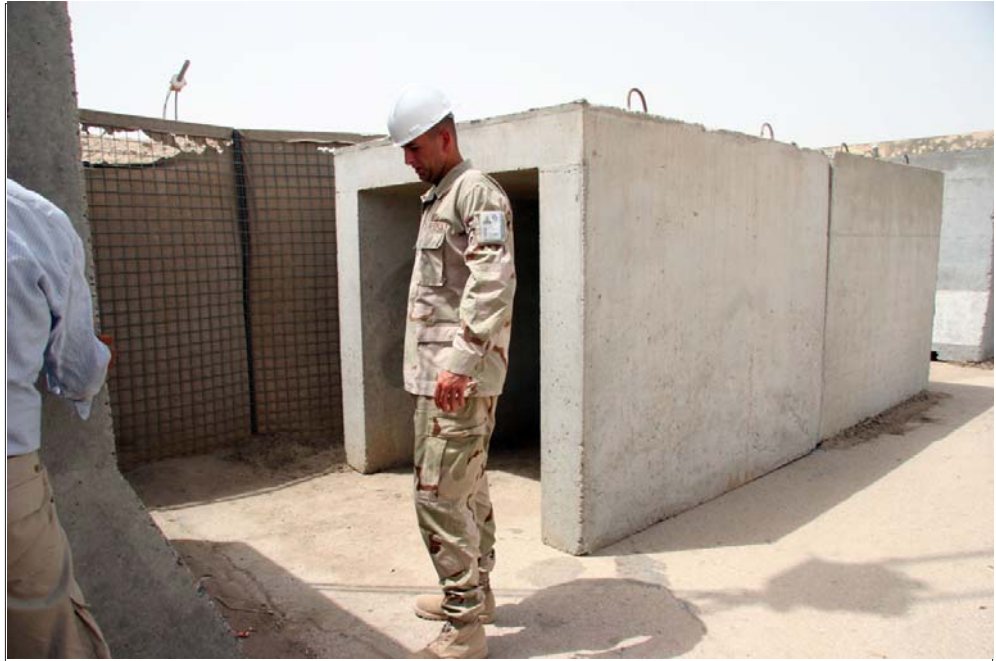
Senior Airman Thomas Ard, 407th ECES, monitors the contractors who are placing a t-wall at one of the entrances to a bunker barrier at the passenger terminal, July 31.
