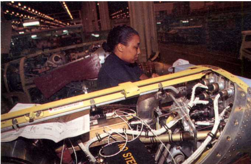
One of the next major steps is adding the engines. The C-130J has four new Allison AE 2100D3 engines that will be eighteen percent more fuel-efficient and will provide thirty-one percent more takeoff thrust. They also turn the transport's most visible new item—a Dowty Aerospace R391 all-composite six-blade propeller. The C-130J shares some technology with modern fighters: two mission computers, power-by-wire technology for the engines and propellers, and head-up displays for both pilots. At left, C. J. Stegall-Evans works on an Allison T56 engine before its installation on a C-130H.
