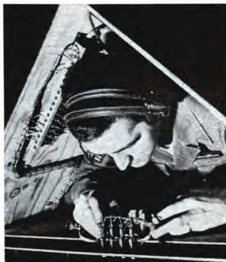
Running on-base communications means getting the job done fast and expertly. At left, an AFCS phone installation man puts the finishing touches on circuitry for a complex intercom system planned by AFCS.
