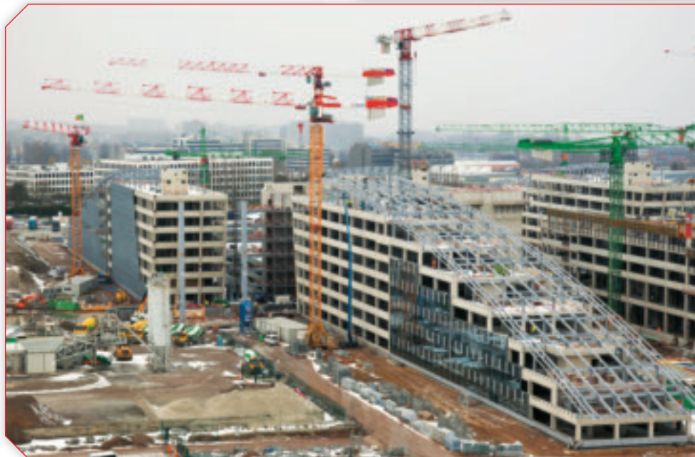
NATO's new headquarters complex, shown here in March 2013 under construction, is right across the street from its current HQ.
